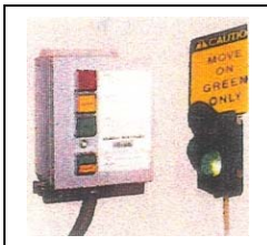
Control box and exterior signal light unit.
